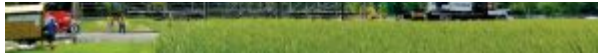
Figure 1. Removal of the bridge from its original location. Courtesy of McCormick Taylor.
